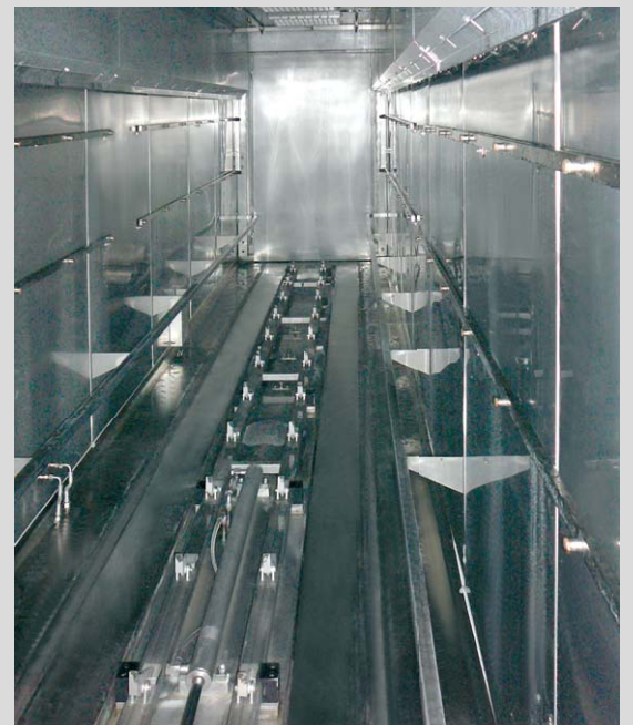
Hydraulic transport system
